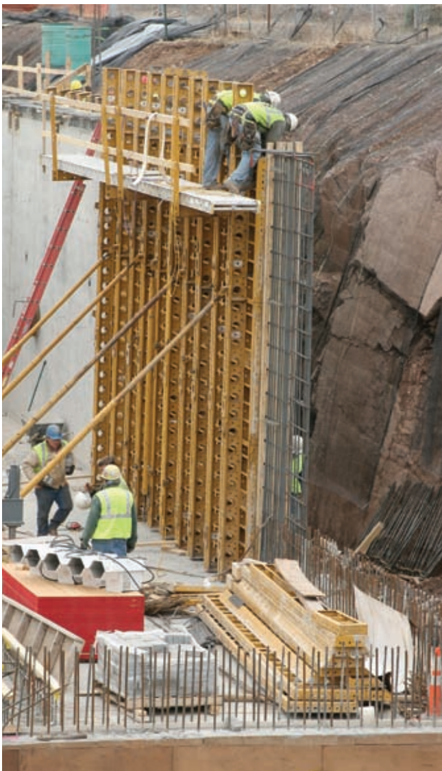
Four overflow storage basins have been built to help eliminate overflows in WLSSD's and the city of Duluth's sewer systems—totaling 4.3 million gallons of storage for excess sewage when capacity of the sewer pipes is exceeded. Up to three more basins will likely be built in Duluth's system in the future to meet federal expectations.
